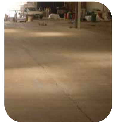
Concrete surface primed using Resichem 503 SPEP prior to application of Resichem 501 CRSG
